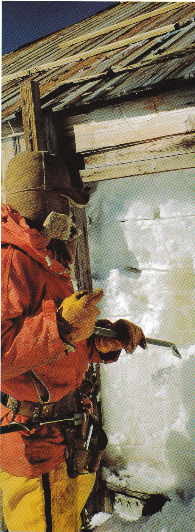
A wall of solid ice confronted team members when they opened the front door to Mawson's Main Hut. The ice was carved into blocks with an electric chainsaw then removed by hand.
