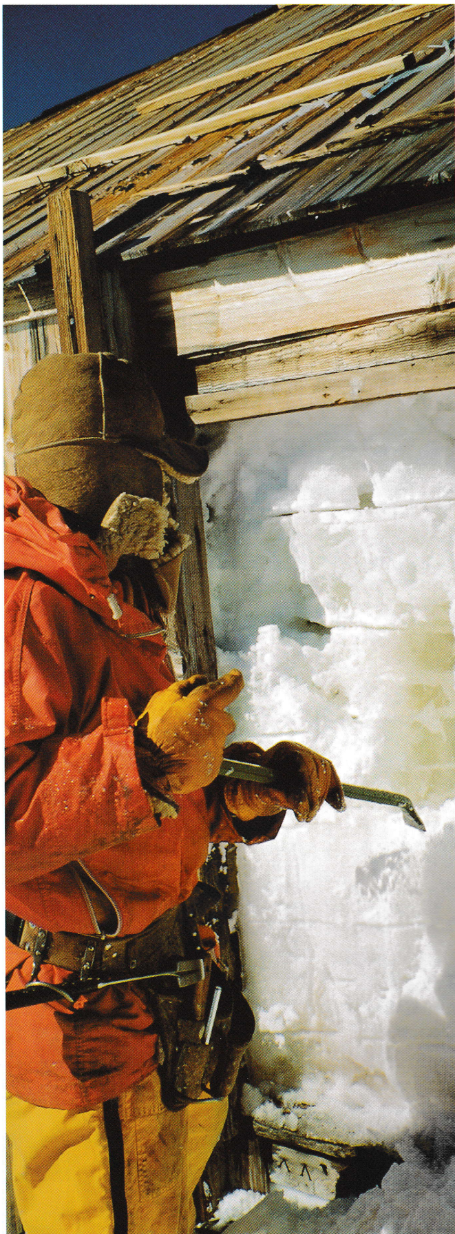
A wall of solid ice confronted team members when they opened the front door to Mawson's Main Hut. The ice was carved into blocks with an electric chainsaw then removed by hand.
