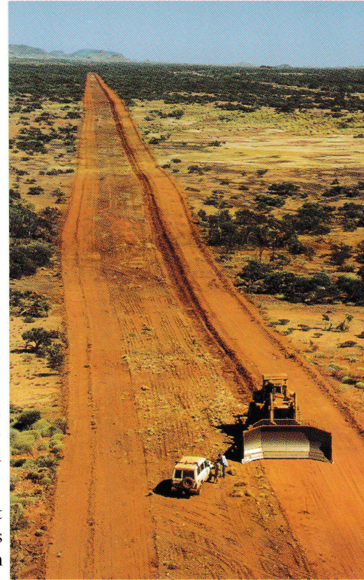
Work is progressing rapidly on WA's new 1,380 km gas pipeline to Kalgoorlie
