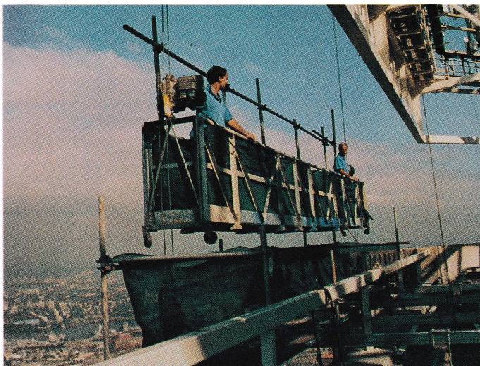
Gavan and his father Ron ride the cradle they worked in each day from the rooftop to the steel structure supporting the new signs
