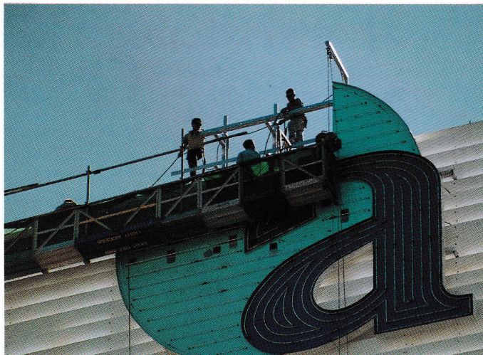
The figures of the workmen are dwarfed by the sign’s size as they work to install the last part of the globe surrounding the first ‘a’
