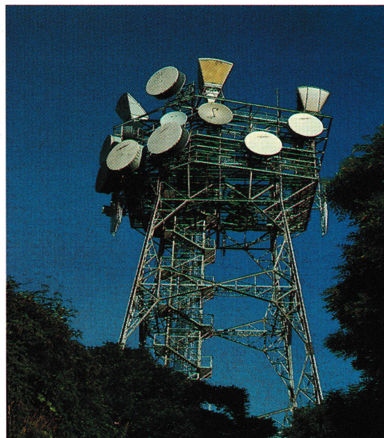
A microwave communications tower
